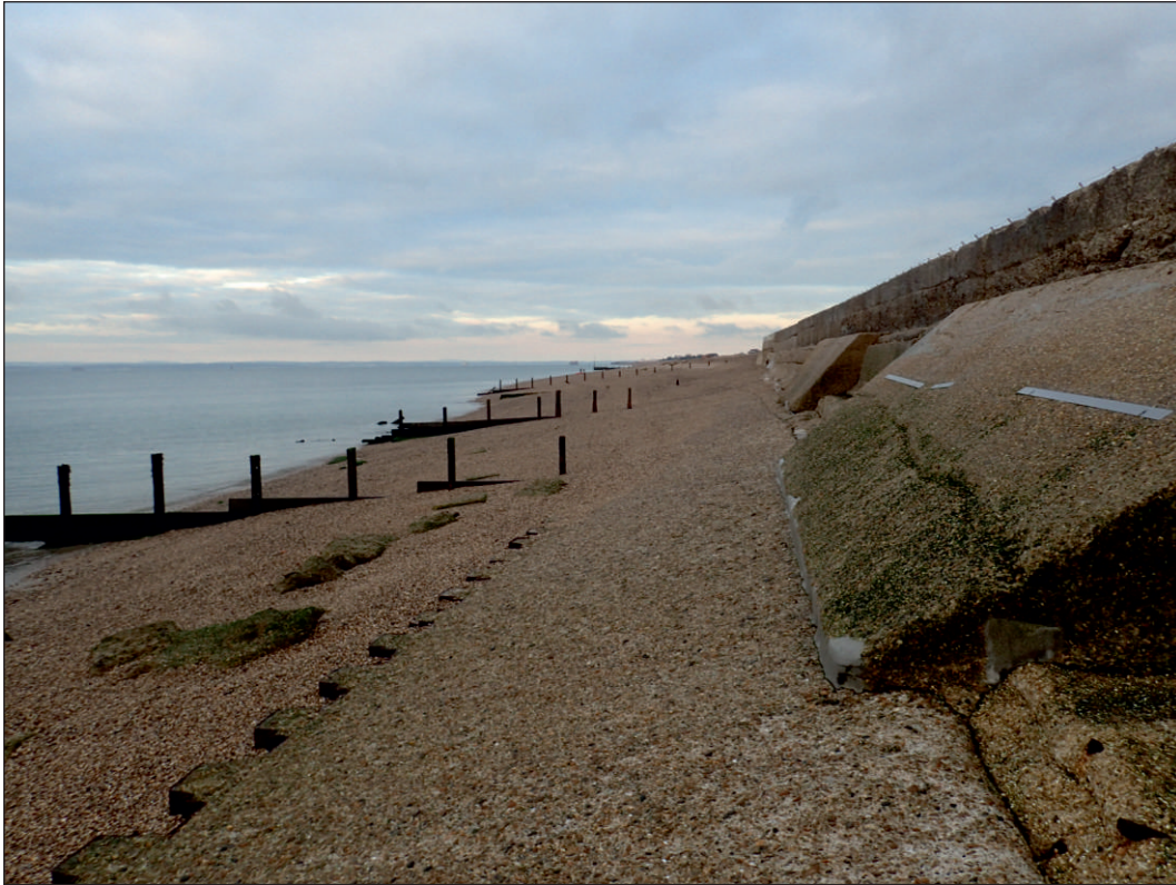
Plate 1: East end of Eastney beach; remains of timber and steel groynes, photograph taken facing west
